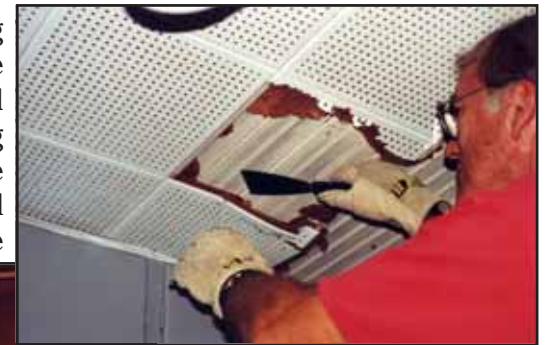
Pete Perenkovich (above and left) uses a pry bar and putty knife to delicately expose beaded board walls and ceilings that date to the 1920s house expansion by Captain Jack DeLysle.
