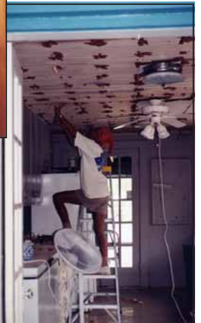
Joyce Heckman (above) and Susie Perenkovich (left) remove nails and staples that held the cardboard ceiling tiles in place. We have Will and Florence Long to thank for covering rather than resurfacing the beaded board. The use of furring strips prevented damage to much of the trim work and protected surfaces until their rediscovery.
